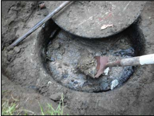
Before - critical failure of septic system with 6 inch thick scum layer
