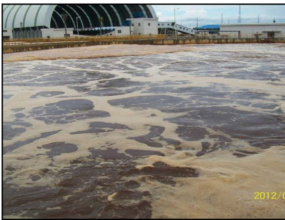
Paper Mill Wastewater Treatment System
