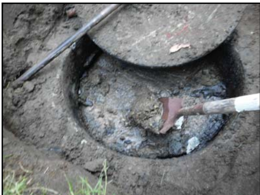
Before - critical failure of septic system with 6 inch thick sludge
