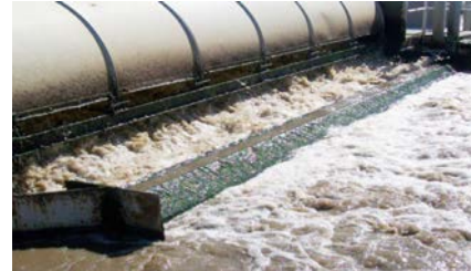
Figure 7: Oxidation Ditch Without Foaming After BIO GENESIS® application
