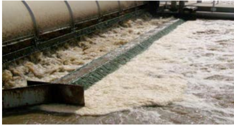
Figure 6: Oxidation Ditch With Foaming Before BIO GENESIS® application
